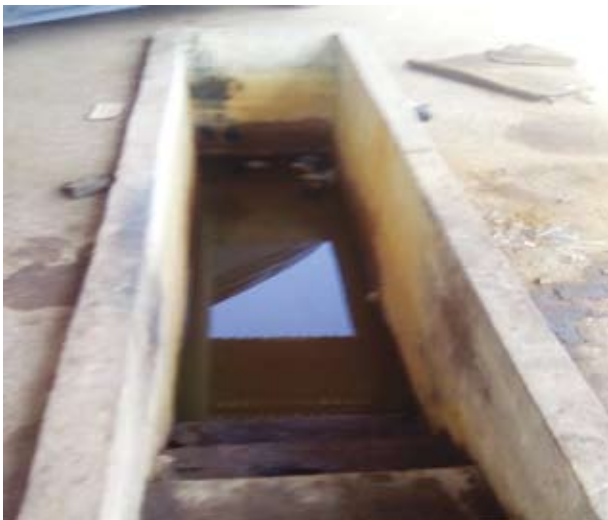
Beneficiaries of the garages are not able to use their service pits because it is always full of underground water.
