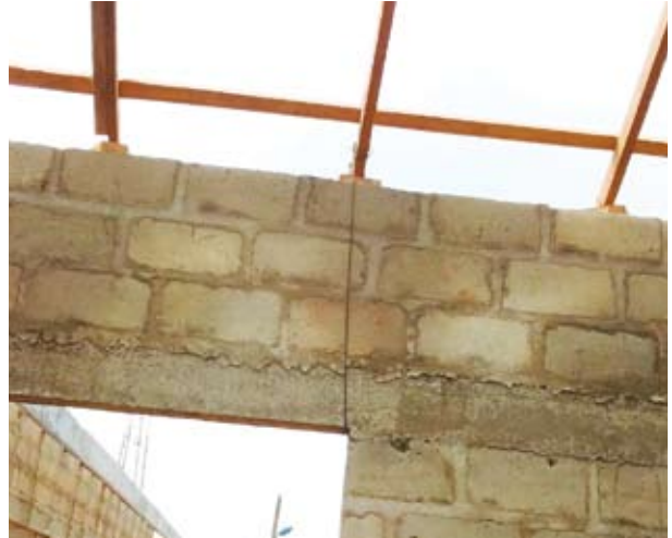
The diameter of the roof hooks is small its functionality is likely to be compromised due to possible corrosion because of exposure to the sea breeze
