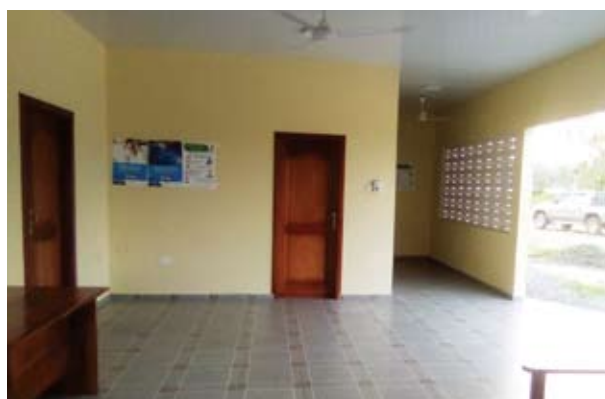
The facility is without fire safety gadgets to give early warning signals of fire and possibly quench the fire in case of an outbreak.
