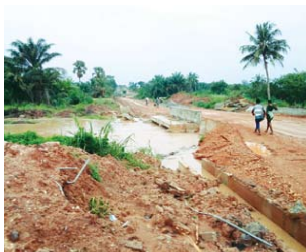
Evidence of inadequate construction signs to communicate to road users.
