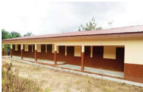
Standardization ought to be informed by trade use to avert post-occupancy modification to fit trade use.
