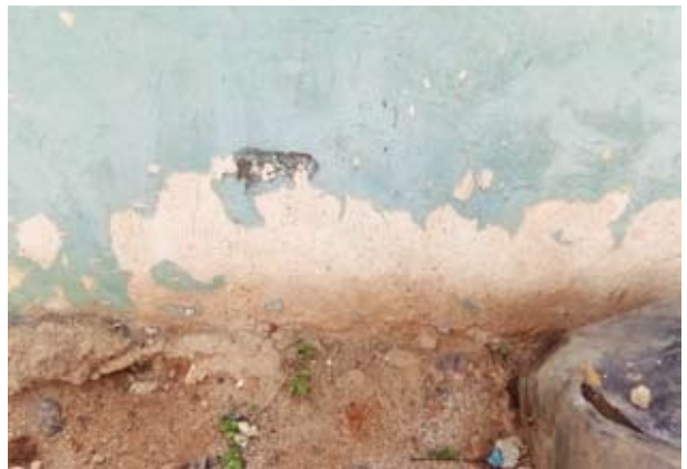
Rising damp on walls due to rising underground water by capillary action. Evidence of not considering the recommendations from the feasibility study at the design and construction stages of the project.
