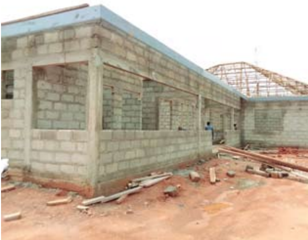
Workers work without appropriate PPEs thus endangering their safety at work.
