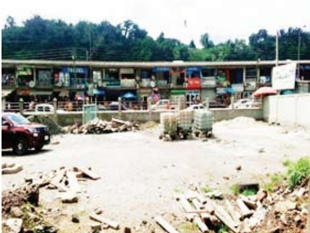
Improper housekeeping at site endangers workers' safety.
