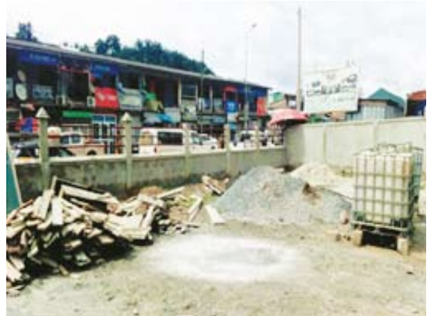
Poor material storage practices on site are a risk to workers' safety
