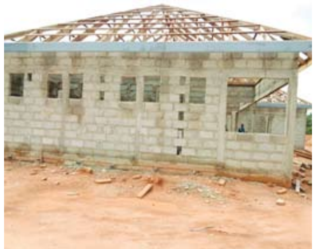
Quality of concrete works could not be guaranteed as payment was based only on the quantum of work done.
