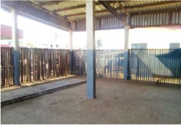
Abandoned garage because the garage is not connected to power source though the owner has improvised to fit trade.
