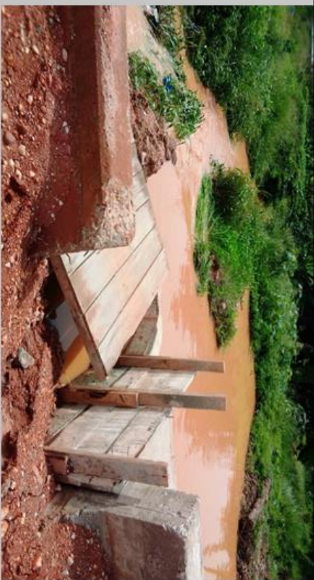
Providing a retaining wall to link the old and the new culverts could avert the incidence of depression due to drifting of the sub-base and base materials.
