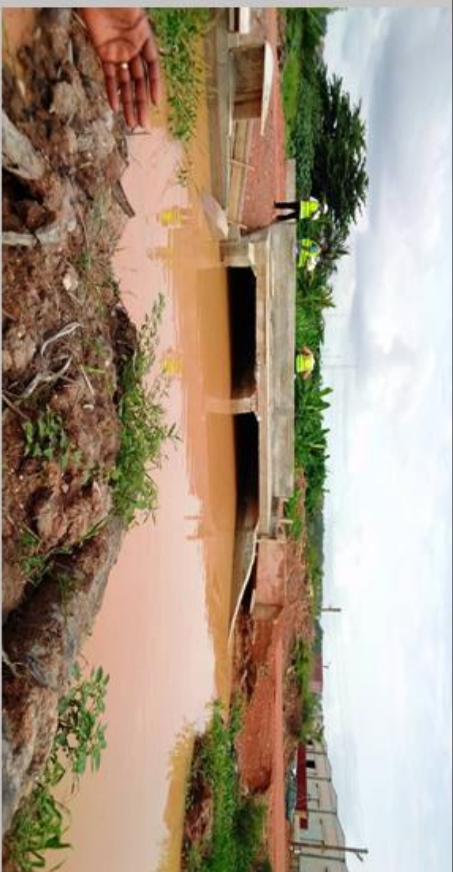
The old and the new culverts could be linked to enhance water flow and avert depression due to drifting of base and sub-base materials.
