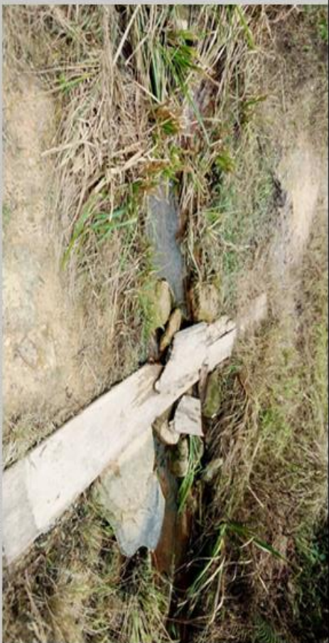
Access to the school needs improvement
