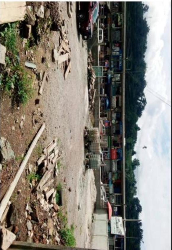
Improper housekeeping at site endangers workers' safety
