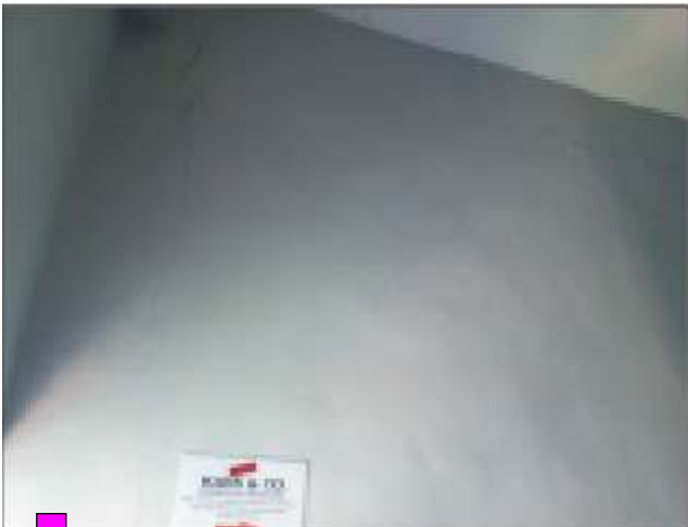
Cracks in walls and leakages in floors at the Library Complex ought to be addressed to avert further deteriorating of the structure
