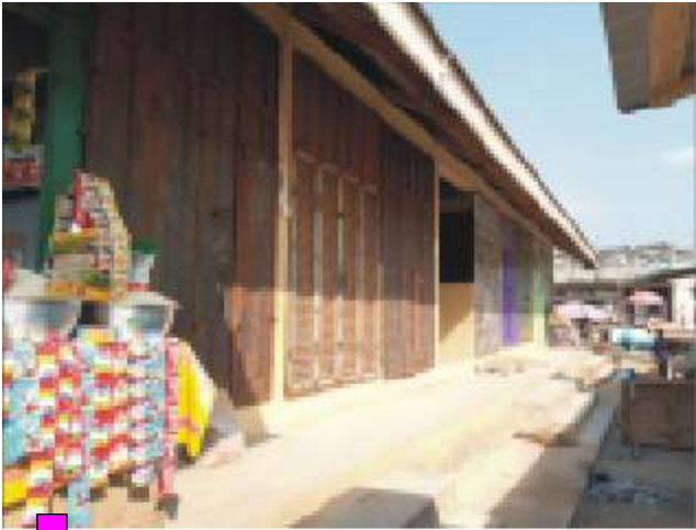
Beneficiaries of the market sheds are converting their sheds into lockable stores, an indication of their needs not incorporated at design stage.
