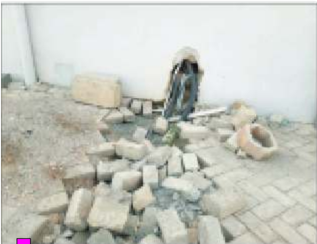
Service hole ought to be made good and paving works completed at the Library Complex
