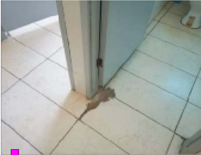
Defective tiles and poor workmanship at the Library complex ought to be remedied.
