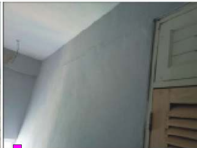
Fittings and light accessories ought to be fixed and cracks remedied.
