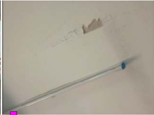
Defective painting due to leakage in floor slab
